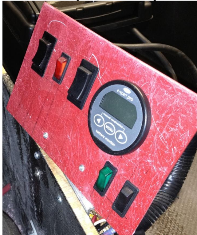
Figure 2 - Control Panel (from left to right switches are number 1-5 respectively)
