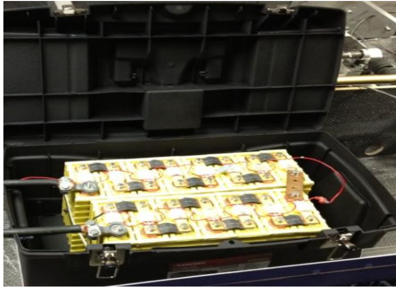
Figure 14 - Thunder Sky LiFePO4 Power Batteries
