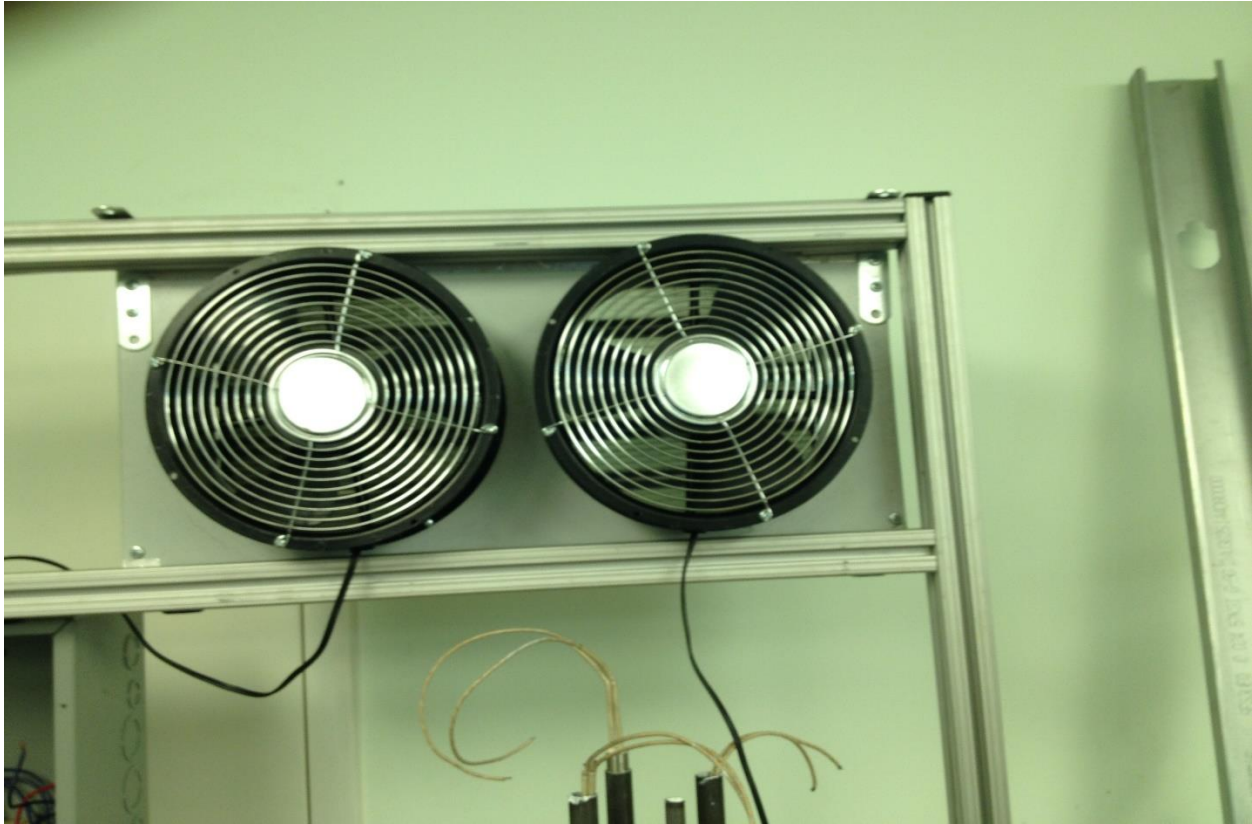
Figure 3. Load with fans attached to 80/20 frame
