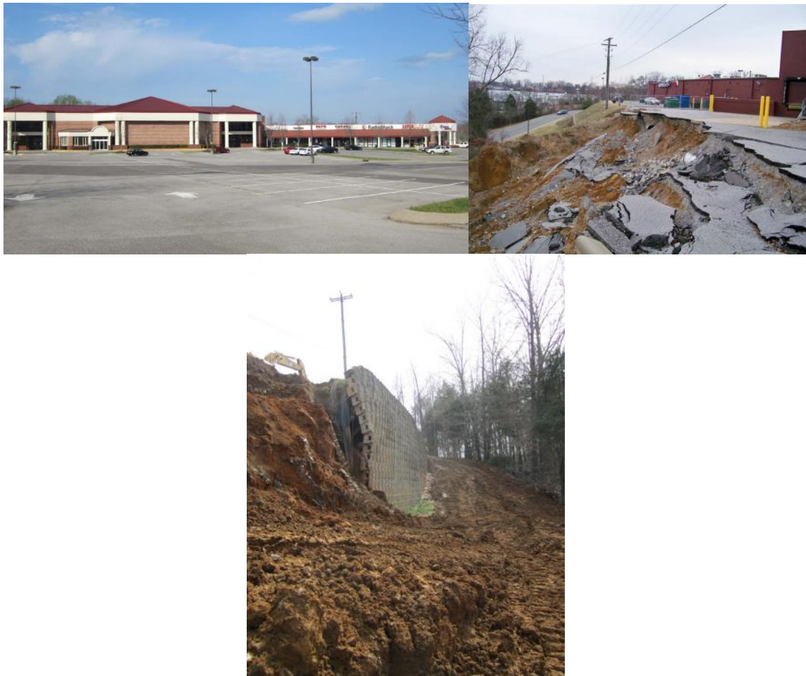
Fig. 2.4: A failure of an MSE wall in Crossgate Shopping Center Nashville, TN (source : http://www.marshall.edu/cegas/geohazards/2012pdf/presentations/S7/1_Geohazards-%20Emergency%20Response-%20Beard%20SNLI )
