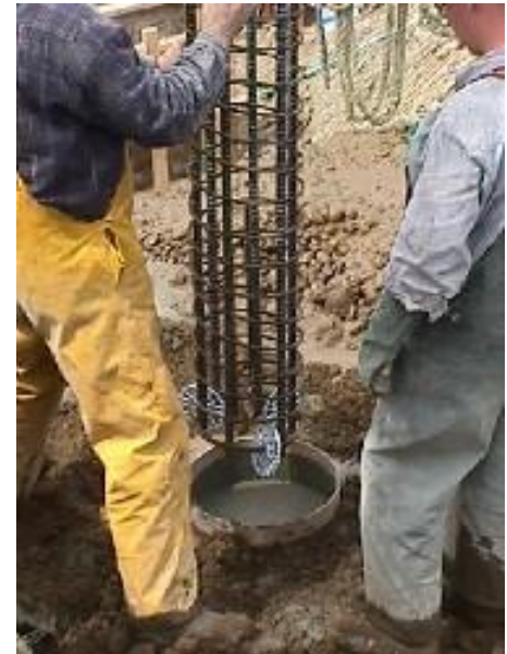
A steel rebar cage is lowered into the hole. The steel is guided all the way down the hole.
